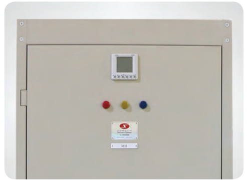
MSB Switchboard with Meter & Lamps
